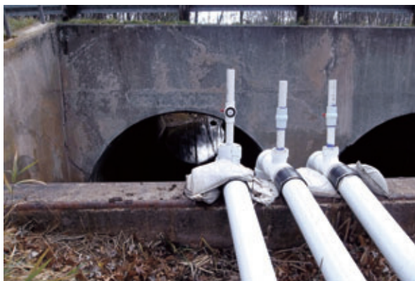
Beecher Lake Dam spillway and culverts under Dam Road (view from north side of dam looking south).
